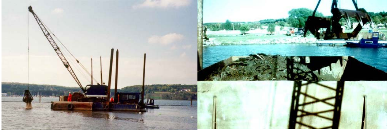
Picture 2: Offloading ramp. Excavator used to transfer wastes from barges to trucks
